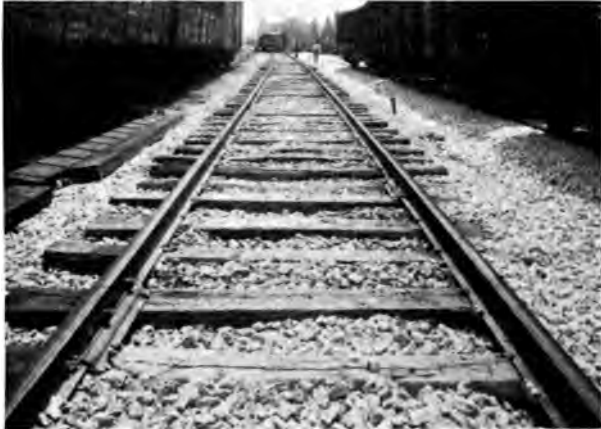
P. & M. Rail Anti-Creepers on the Chicago & North-Western Railway near Deering, Illinois
